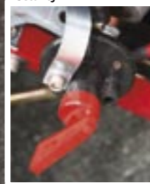
Hidden battery cut-off switch can disable the Mini quickly for safety or security
